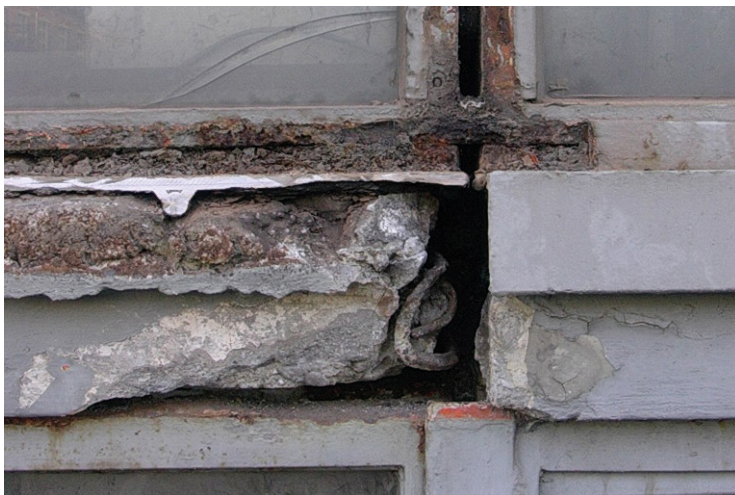
Figure 2 Exploratory investigation of deterioration on the north façade at an expansion joint.
