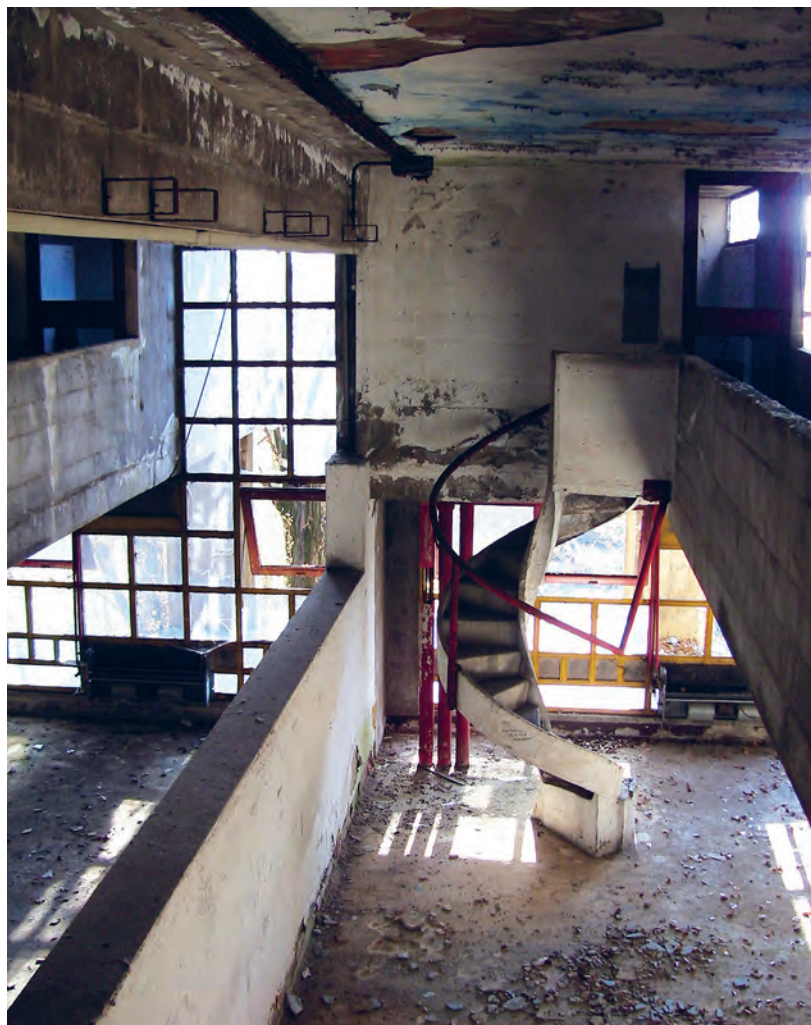
Figure 3. View of the present condi- tion of one resi- dential dormi- tory.
