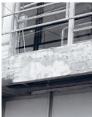
Figure 9. Decay in the external reinforced-con- crete structures: rust spots, crack- ing, delamina- tion, spalling.
