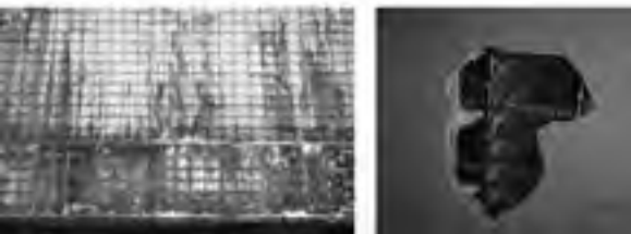
FIGURE 3. Conservation problems at the Institute of Mycology. East façade and the plasterboards covering the glass breeze-blocks. © Fernando Diniz Moreira.
