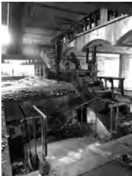
FIGURE 3. St Peter's Seminary, view of interior damage, 2015. © Avanti Architects.
