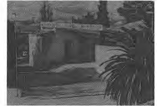
The external portico with the original pergola that collapsed during the 1980-81 earthquakes
