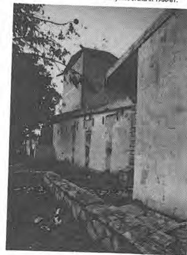
The southern elevation of the church shows the serious damage due to the seismic events in 1980-81.
