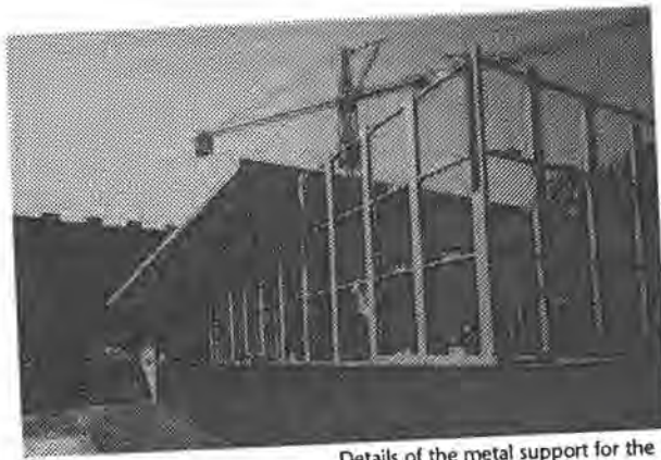
Details of the metal support for the green Alpine marble. Main entrance (April 1985)
