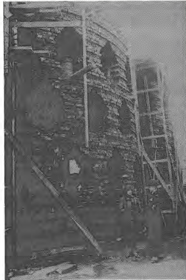
Rationalisation of traditional construction techniques: Melnikov house under construction, Moscow 1928, the architect and his wife on site.
