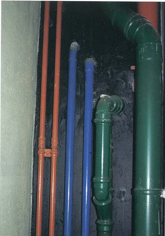
The staircase is equipped with a shaft for utilities. Every colour corresponds with a certain function. (The Renaat Braem house (1958), by Jo Braeken & Tom Lenaerts, p. 92 - p. 94)
