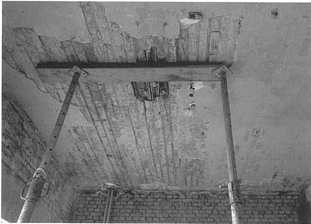
Detail of the 'granilis' plasterwork with starting joint and crack. Photo: Patrick Robyn.
